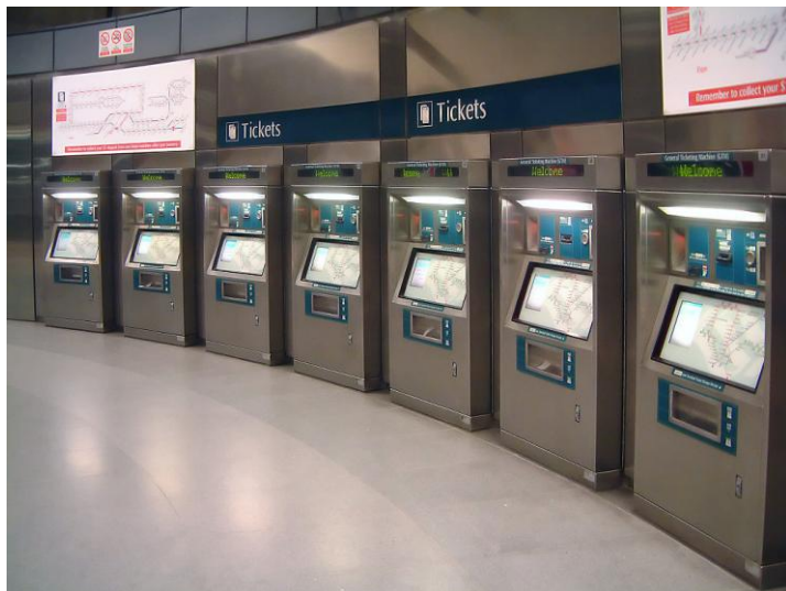
Automated Fare Collection Systems
